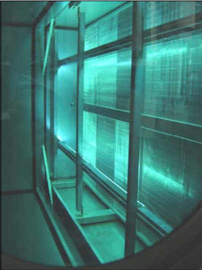
UV lights shining on the down-stream side of a cooling coil
